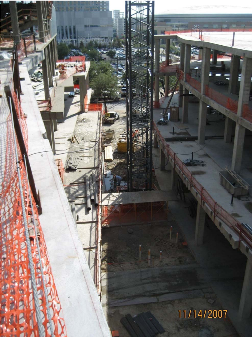
LEFT PHOTO - BLOCK 274 VIEW OF EXTERIOR PLAZA FROM ROOF OF HOUSE OF BLUES.
