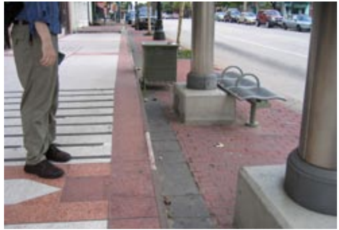
The north sidewalk across the street is not ADA accessible.
